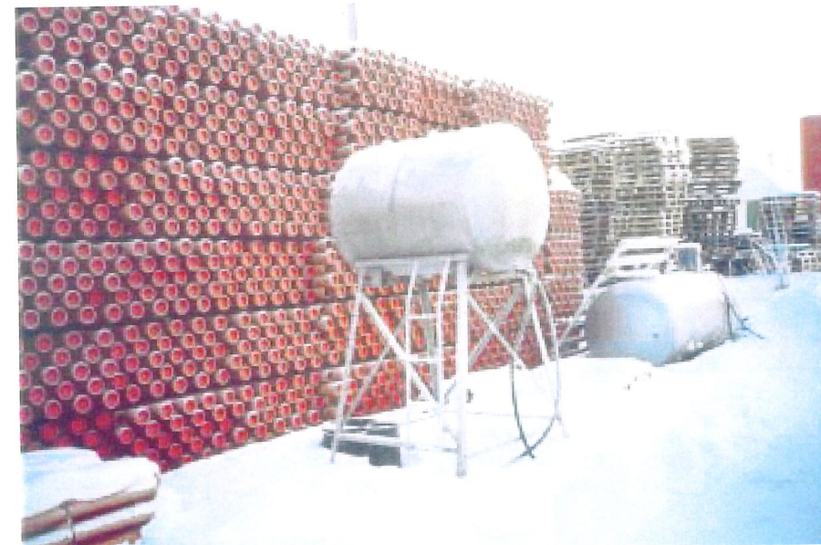
The two AST's for diesel oil
